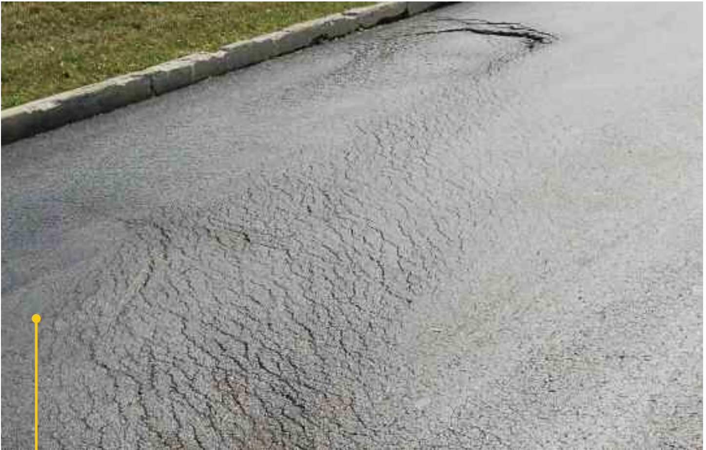
Slippage failures are caused by a lack of bonding between asphalt layers.
