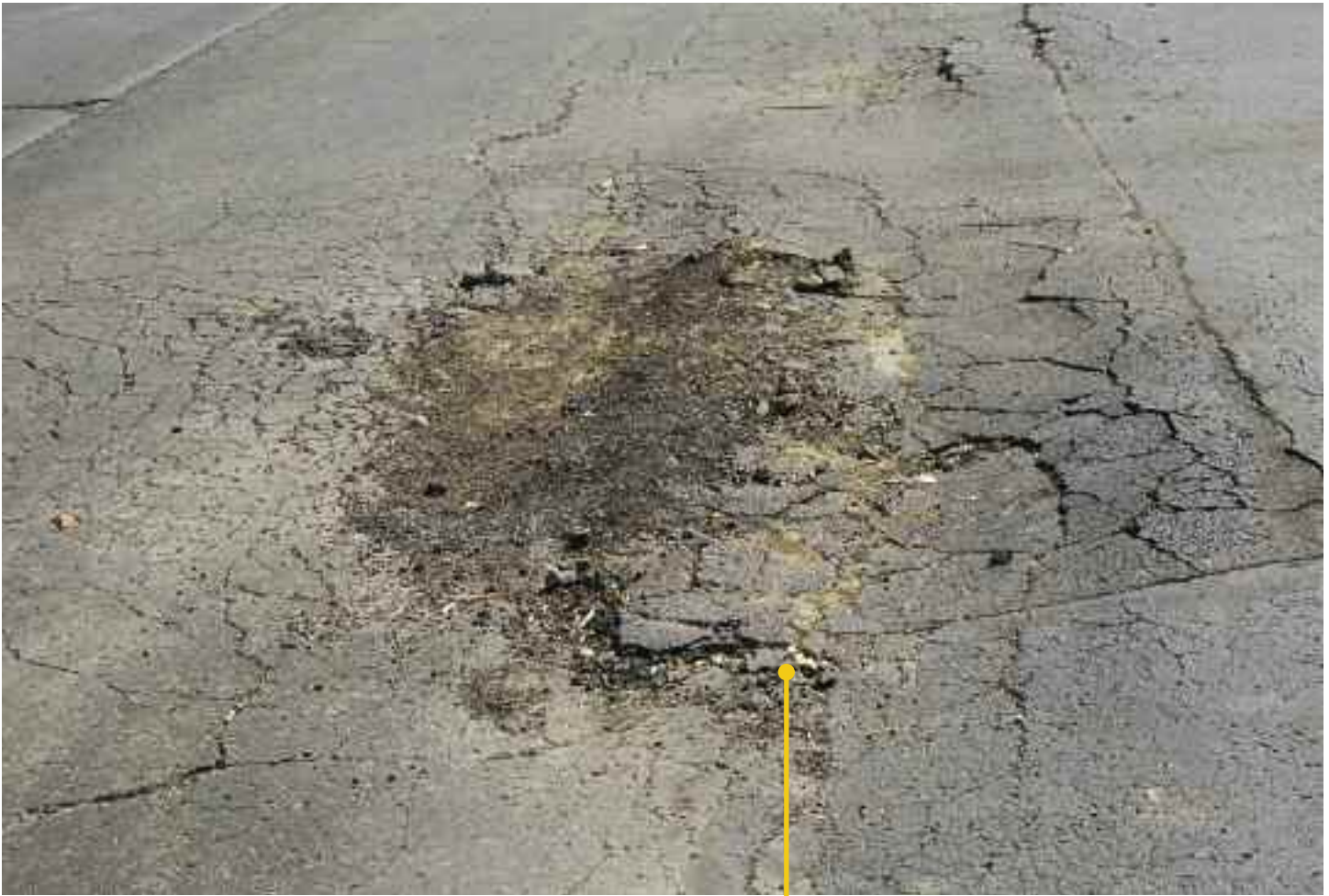
Many pavements fail because the asphalt is simply too thin to carry the loads.
