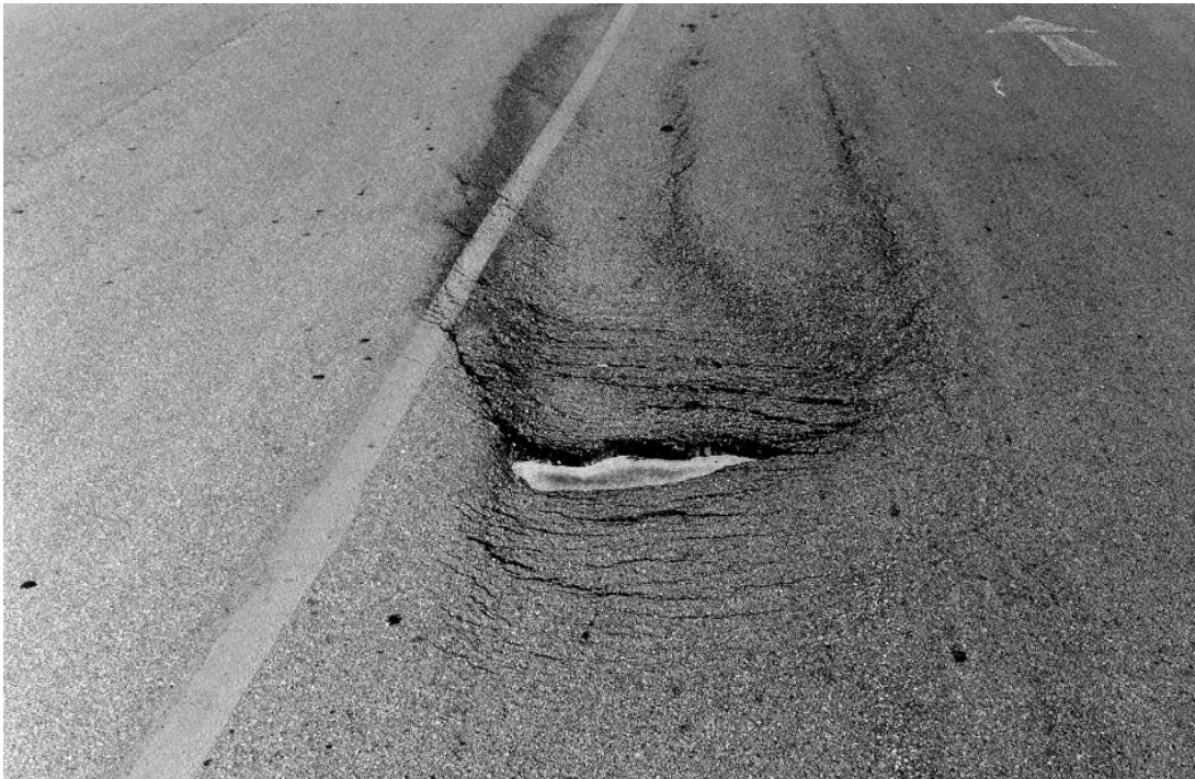
Figure 1. Slippage failure due to poor bonding of pavement layers.
