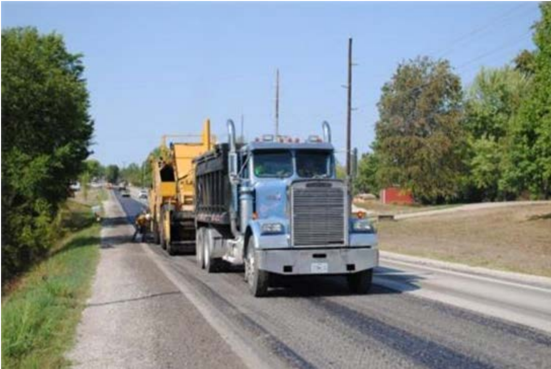
Figure 4. Pavement displaying tack coat which has tracked off the surface.
