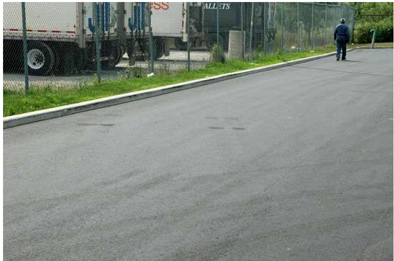
Indentation left from parking of trucks on freshly laid pavement
