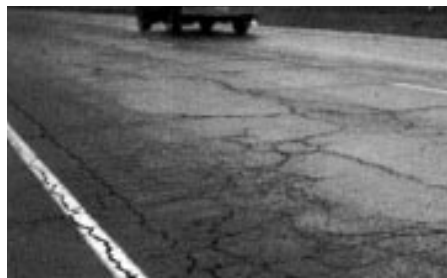
Figure 4. Alligator (fatigue) cracking
