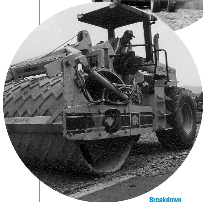
Breakdown compaction after rubblizing with the Multiple-Head Breaker was done with "Z" roller.
